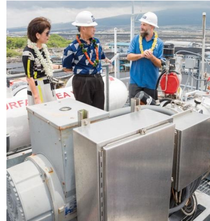
The Governor of Hawaii, David Ige, and his wife Dawn, discuss OTEC with Makai engineer Mike Eldred on the top level of the Makai OTEC plant. The turbine-generator is visible in the foreground.
